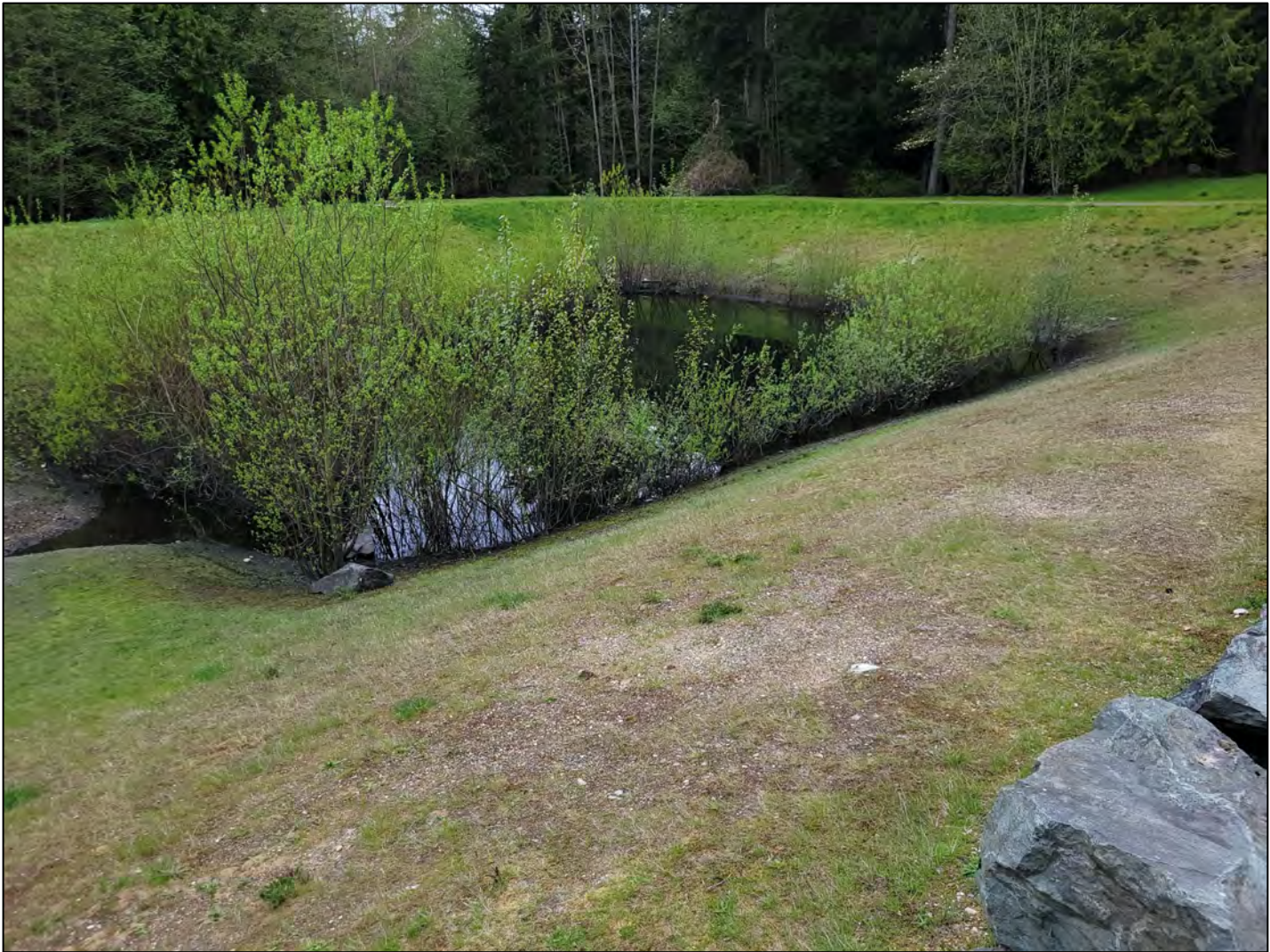
WSDOT stormwater pond looking generally northwest. Note standing water and young trees at bottom of pond.
